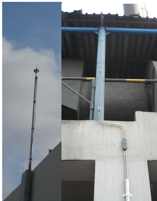
Fig. 5. Early streamer emission lightning rod and grounding conductor sample of new lightning protection system
