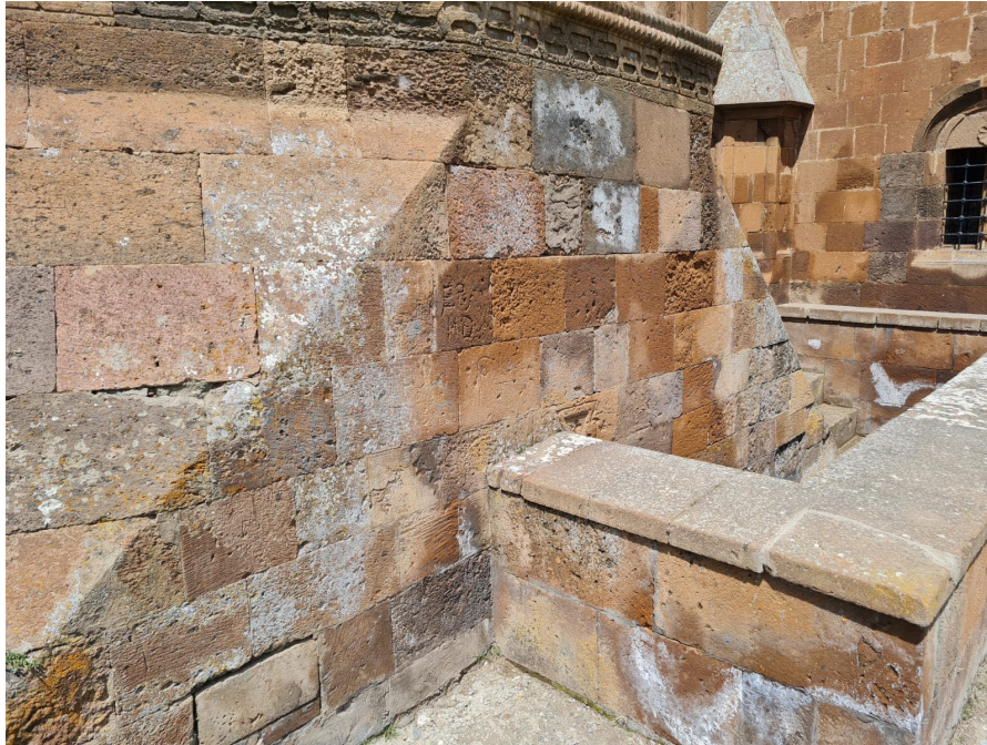
Fig. 5. Efflorescences in the capillary region
