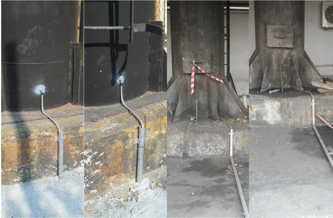
Fig. 6. Grounding of boiler chimneys
