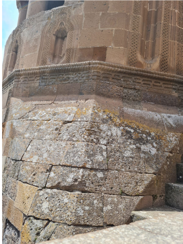
Fig. 3. Deterioration types observed in the monument (missing part, crack differential erosion, lichen deterioration types)
