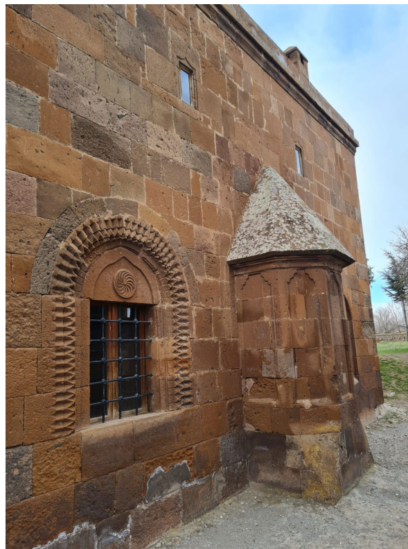
Fig. 4. Deteriorations due to capillary action in the monument
